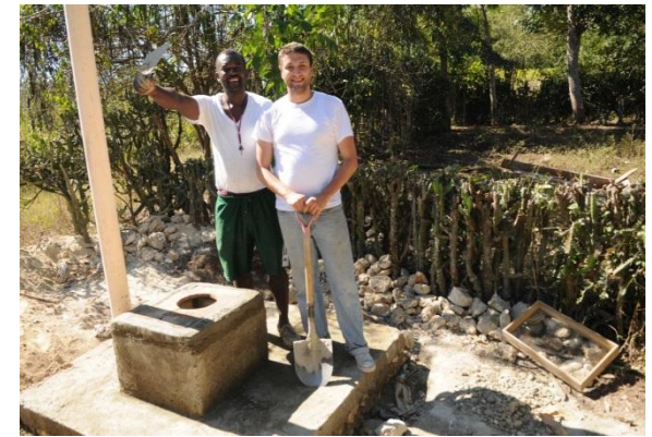
Engineer Benjamin Castleberry and Jacsonville community leader Gabriel Thelus work on building a latrine
