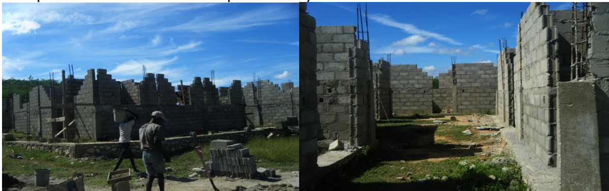
Construction is ongoing year-round by local workers to build the first medical clinic in Jacsonville, Haiti.
